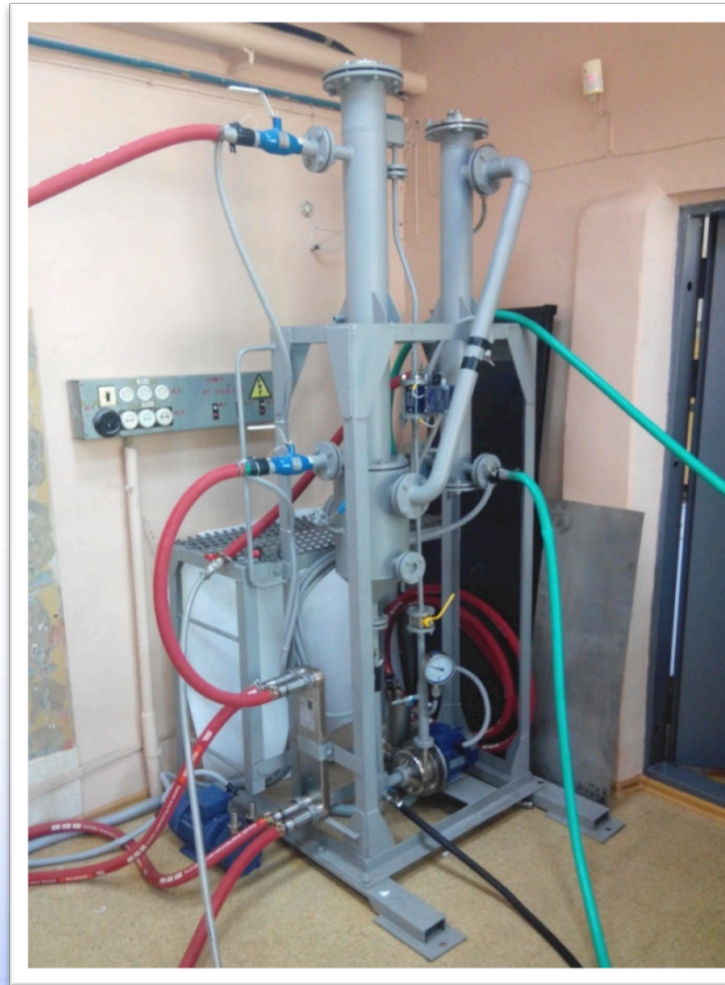
The installation with capacity of 20 kg/h of desalinated water
